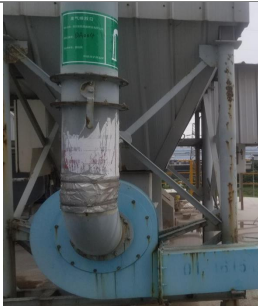
细焙料仓收尘尾气G1-3排气筒DA014
