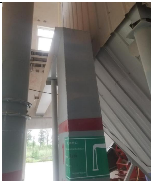
篦冷机下料尾气G1-6排气筒DA028
